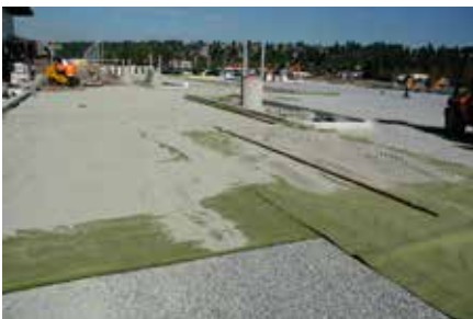
7. Inbitex® is placed followed by the 5 mm clear crushed open-graded Bedding Course .
