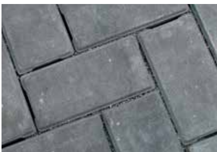
13. Close-up view of the joints with AP Engineered Joint Stabilizer applied before final compaction.
