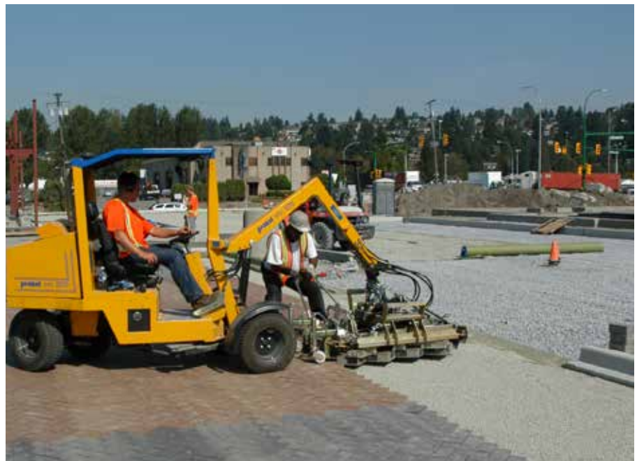
9. AquaPave® is placed using mechanical laying equipment, this can increase production to 8,000-10,000 sq. ft. per day with a standard crew.
