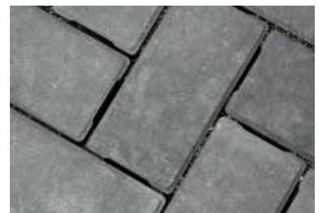
15. Close-up view of the joints with AP Engineered Joint Stabilizer applied after final compaction.
