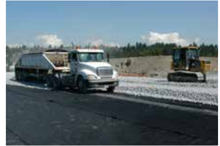
3. Clear crushed open-graded aggregate lower Sub-base is placed, followed by grading and compaction.
