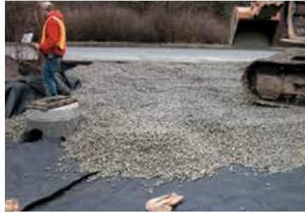
2. Placing and spreading of the clear crushed open-graded lower Sub-base aggregate without wrinkling or folding the geotextile.
